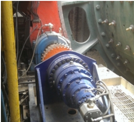
Ball Mill Inching Drive
